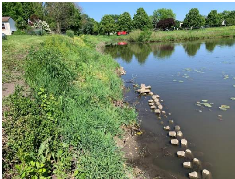
Figure 2.4 Category B – Existing A-Jacks Enforcement, 6-N
